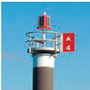
SLC600 installed at Gladstone, Queensland
