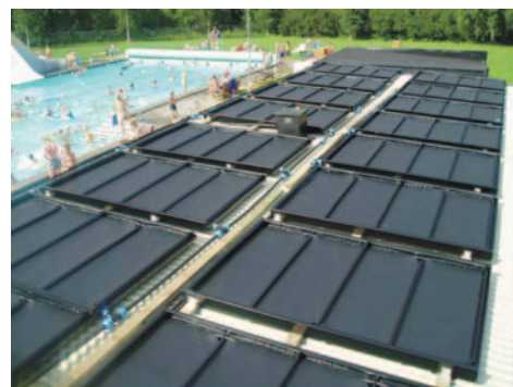
Public pool in Skellefteå, Sweden with 65m 2 solar collectors. Heats the pool and pre-heats tap water.
